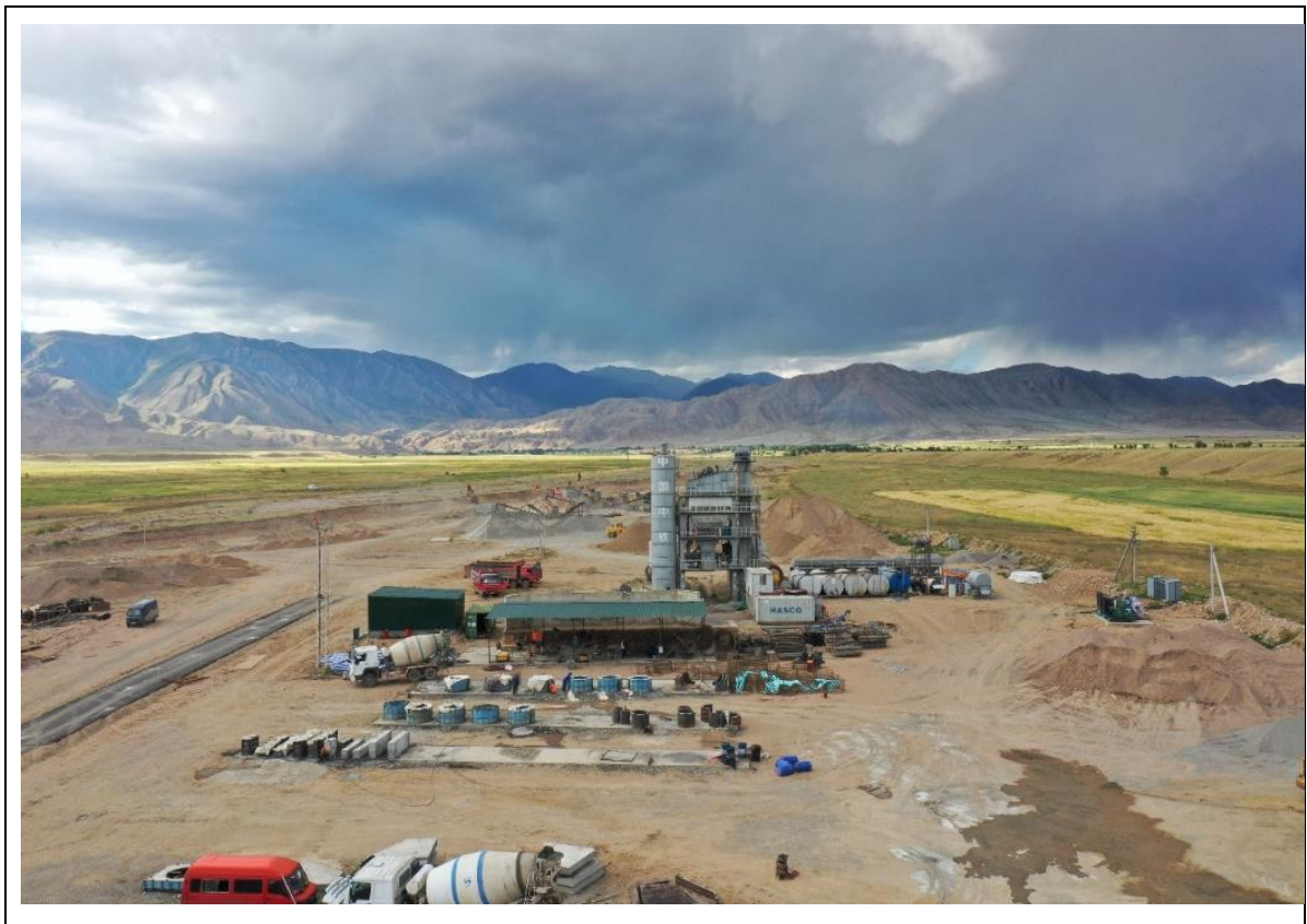
Figure 10 Asphalt plant at the production site.
